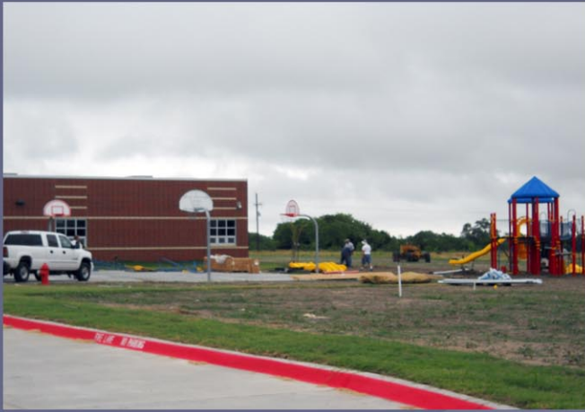
The new playground equipment is being erected next to the exterior basketball court.
